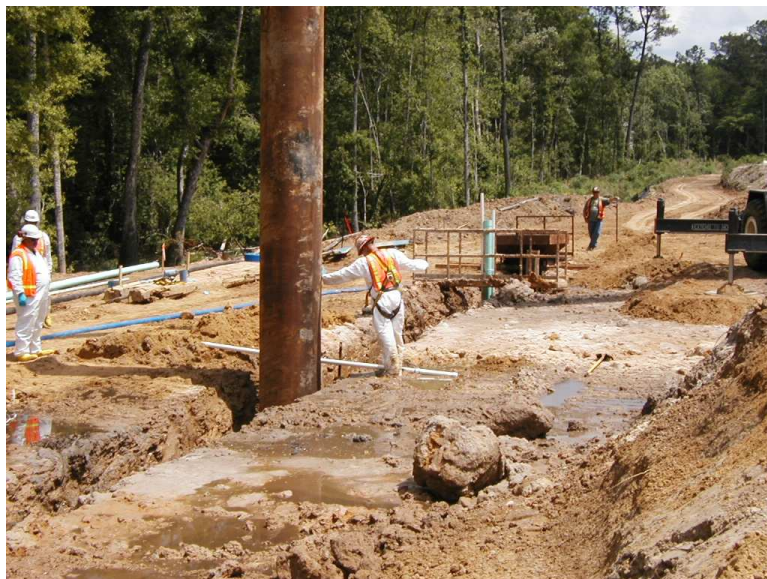
FIGURE 4: Installing end stop in deep trench (note well and tremie in background).
