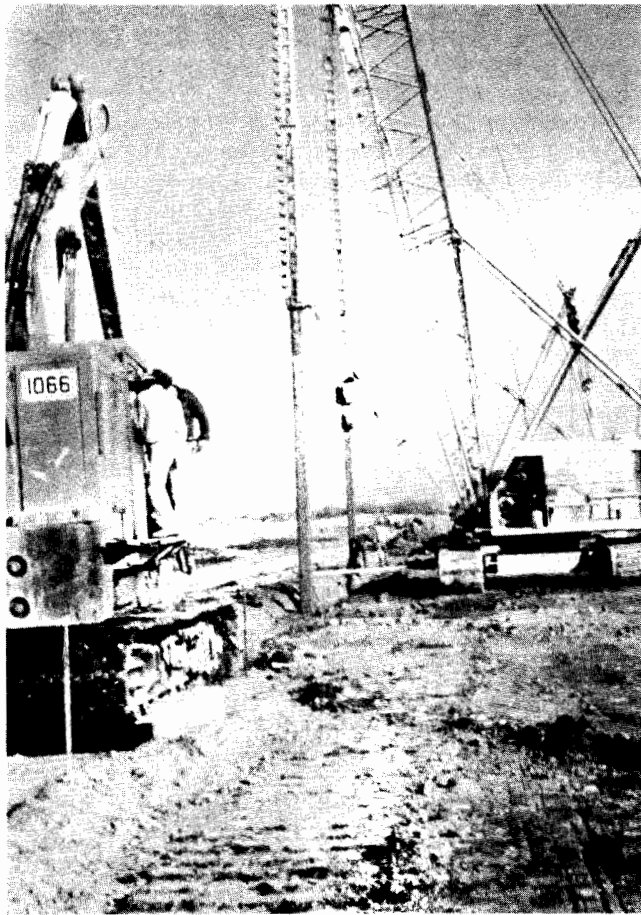
Fig. 10. Two kelly-guided clamshells excavating deep portion of slurry trench. Initial 50-ft depth being excavated with modified backhoe in foreground. Braidwood Power Station, Ill.
