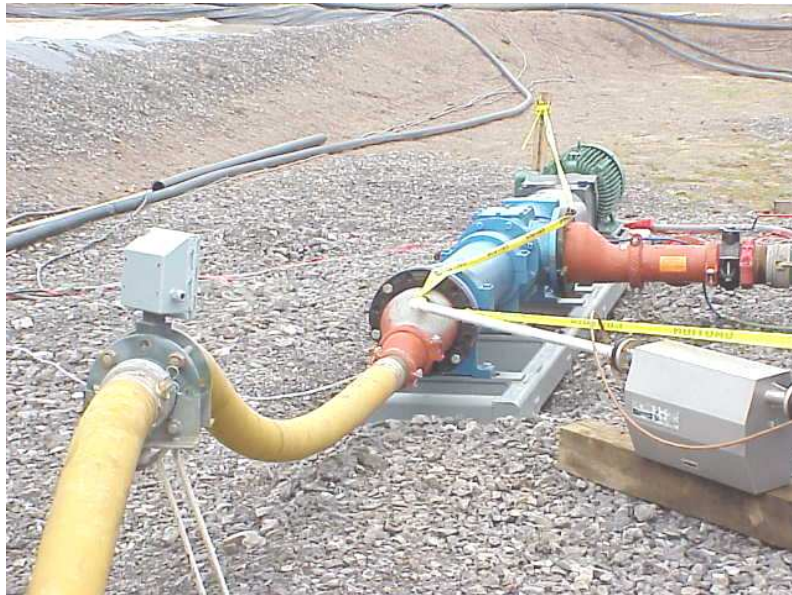
Figures 6. Pumping unit with density meter to the right and flow meter to the left.
