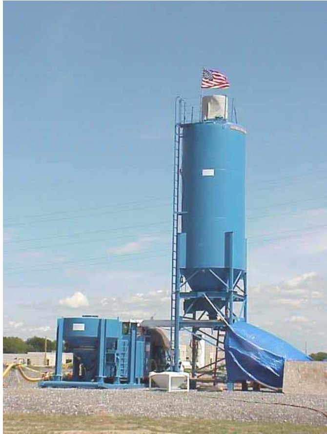
Figure 5. Grout mixing plant
