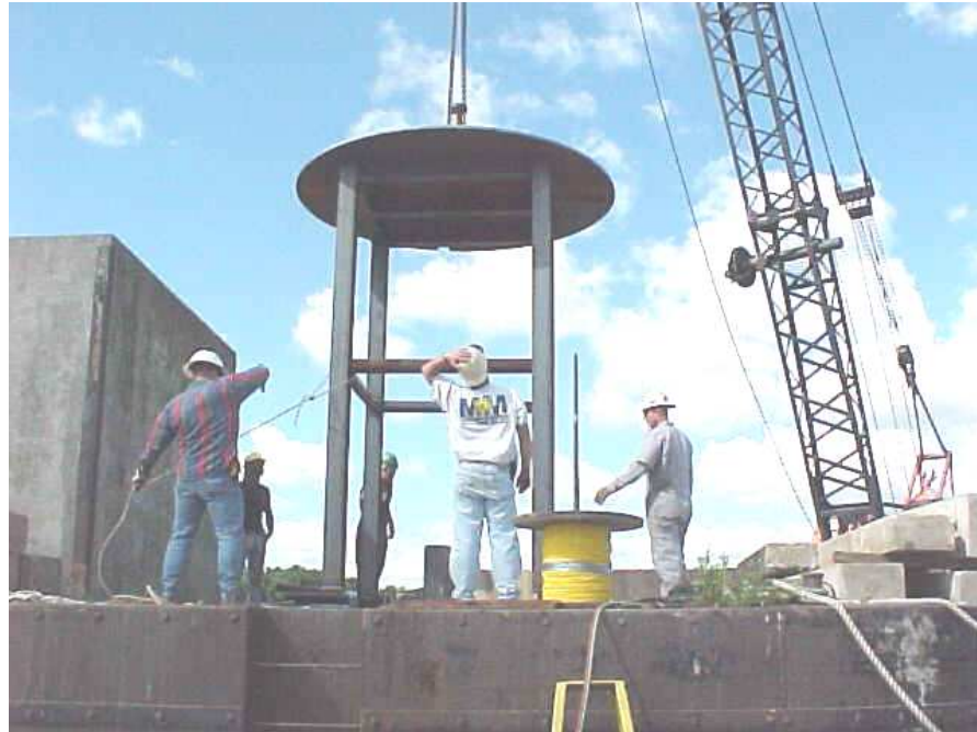
Figure 4. Placing the steel “stool” in the river shaft in preparation for the tremie seal
